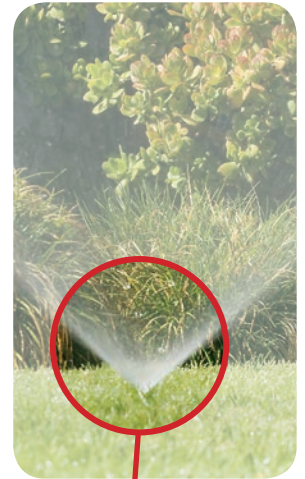
Lawn Irrigation System
